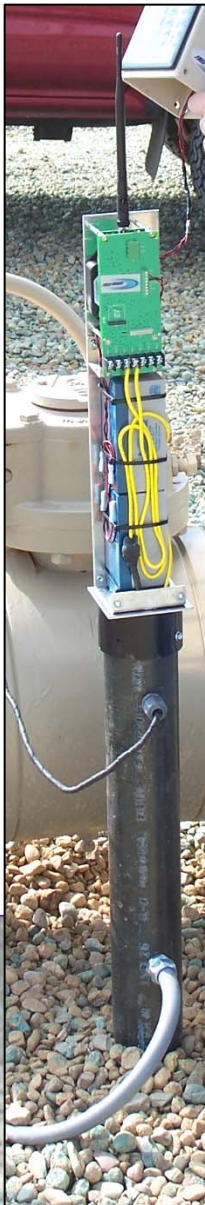
FGRCP LineMarker Test Station
